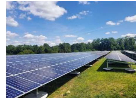
3MW Solar array at former landfill at the Municipality of Princeton's River Road facility.
