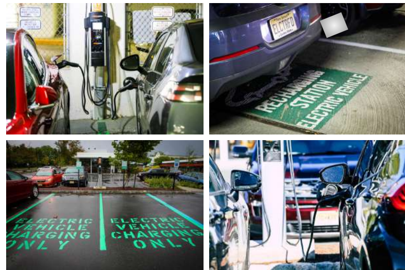
Level 2 public EV charging stations are currently located in Spring Street Garage, Chambers Street Garage and at the Princeton Shopping Center. Preferred locations for future charging stations are workplaces and near public transit.
